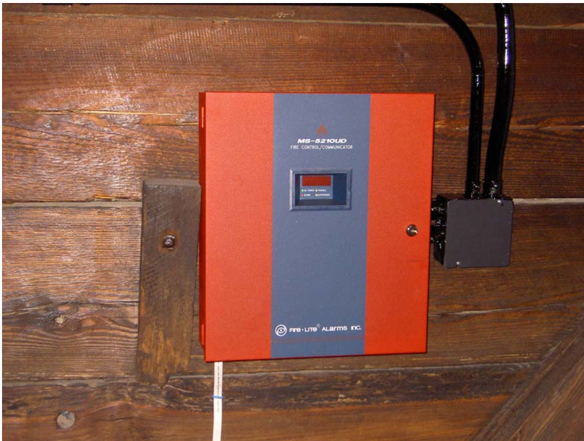
Photo of Fire-Lite Control Panel
